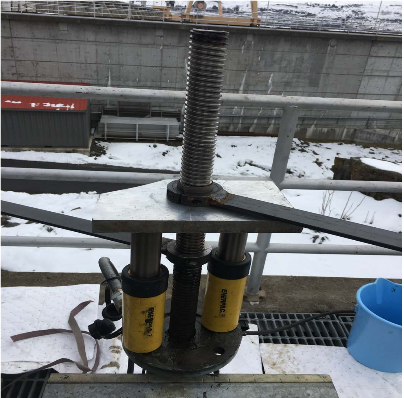
North fishladder flow control diffuser failure. Maintenance improvised manual control system.
